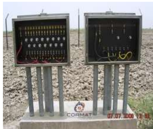
Anode and Cathode Junction Boxes- ICCP System
