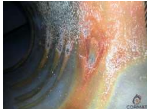
Internal Pitting corrosion in a 26 inch dia. CS Pipeline at 6 'O clock position
